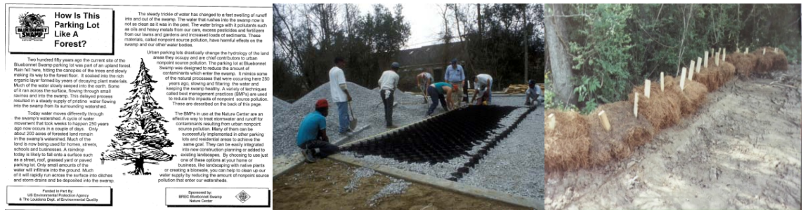
From Left: “How is this parking lot like a Forest” signage explaining BREC’s innovative storm water drainage parking lot design. Construction sites showing BMP’s being used to reduce impact.
